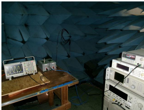
CE102 Signal Path Check
